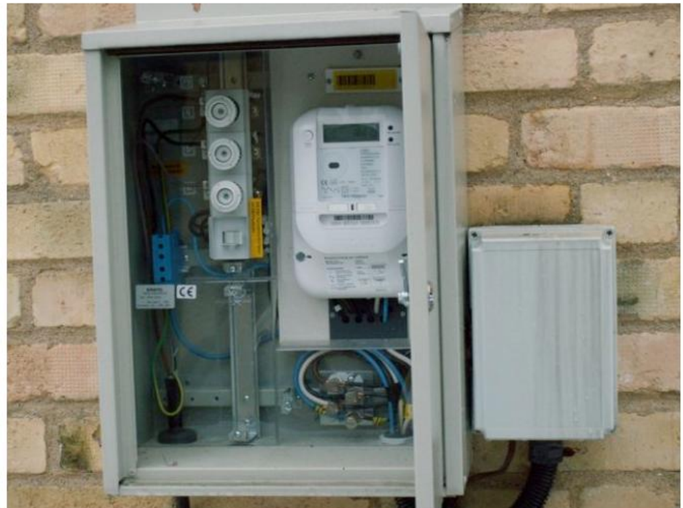
The E.ON filter is the box mounted on the wall to the right of the Lindblom family's electrical meter.
